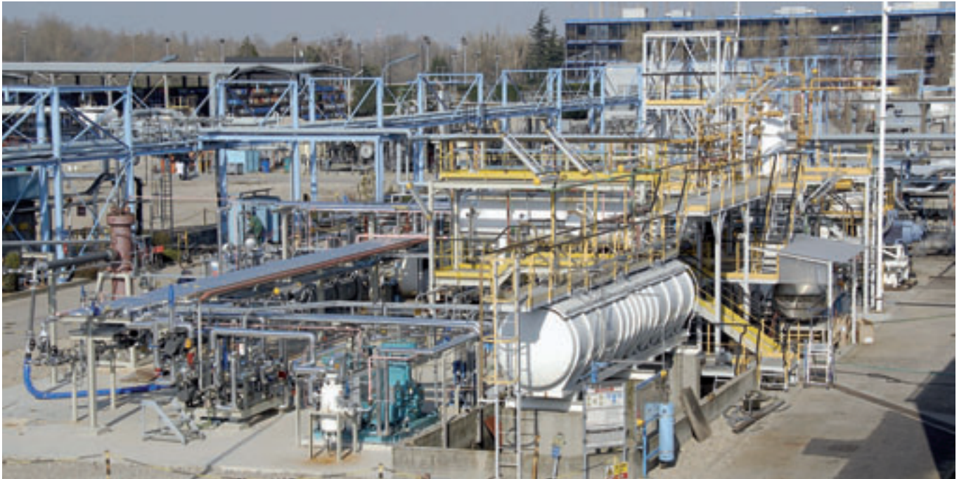
GOwSP gas-oil-water separation platform at Lyon site.
