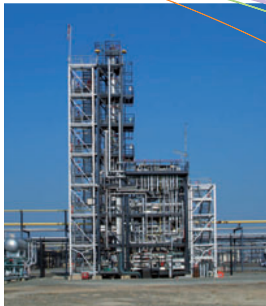
Sprex ® demonstration unit at Lacq using the process developed jointly by IFP Energies nouvelles, Total and Prosernat.
