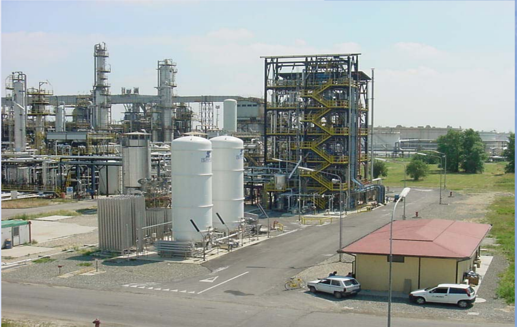
ENI – IFP Pilot Plant (150 kg/h) in Sanazzaro ENI refinery
